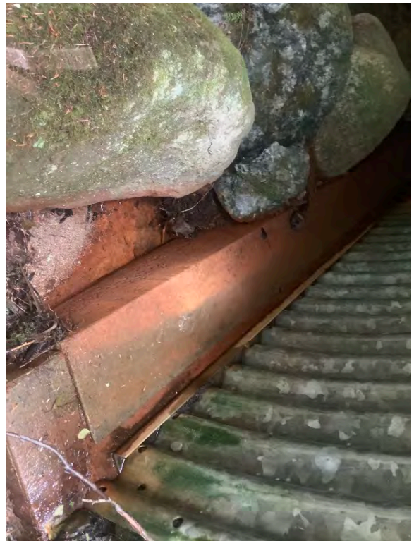
Footing - typical scour
